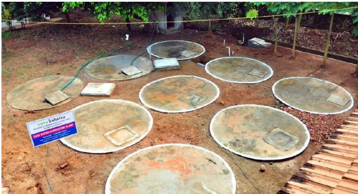
Systematic Rain Water Harvesting, and Bore Well Re-charging system capable of collecting 1.5 Lakh Litre of rain water is operational in Yuvakshetra
