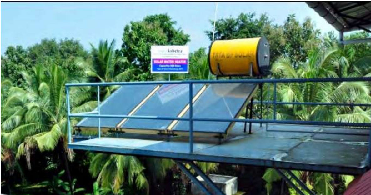
Solar Thermal Water Heating Systems (3 x 100 LPD) capable of raising water to 85°C Addition of Steam Cooker in hostel kitchen saves lot of fuelwood
