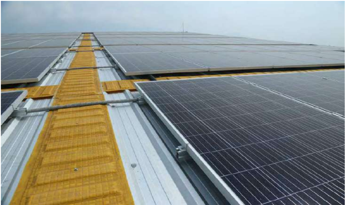
Jubilee Block at YIMS has 60 kW of SPV The energy is fed to the KSEBL grid and YIMS draws power from its existing connections
