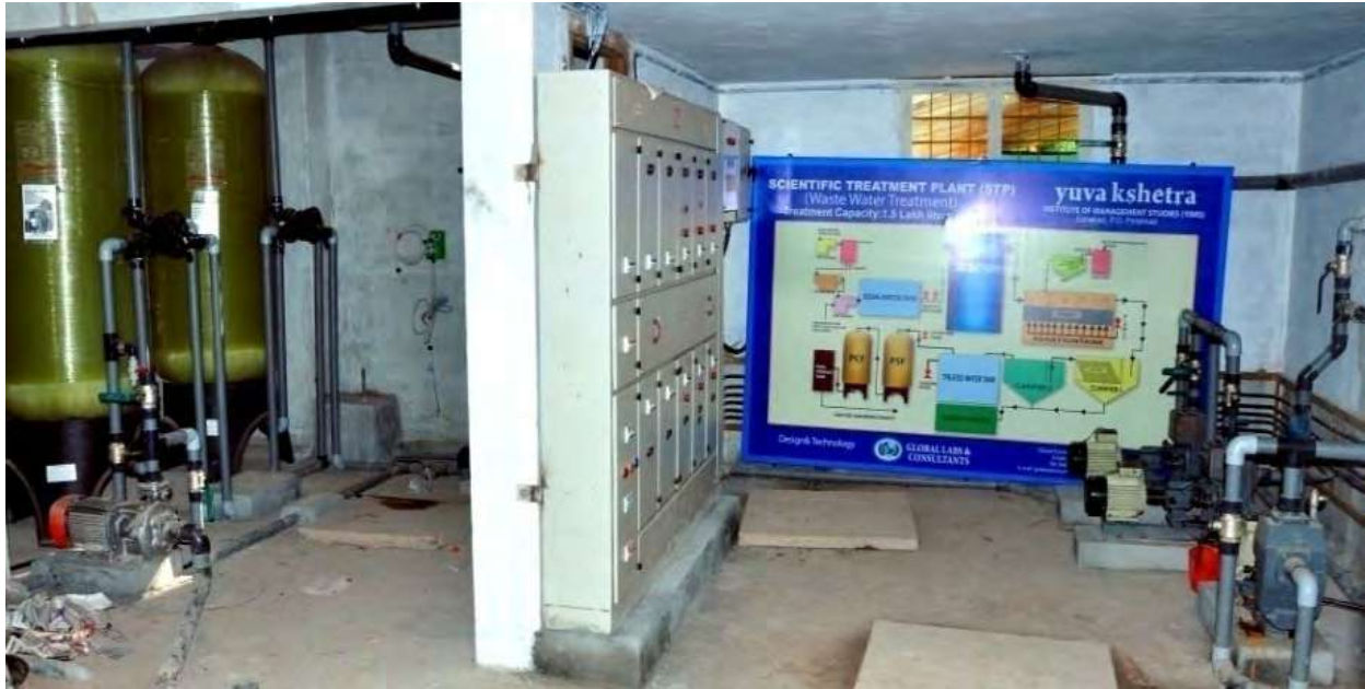
Waste water Treatment Plant at Yuvakshetra
