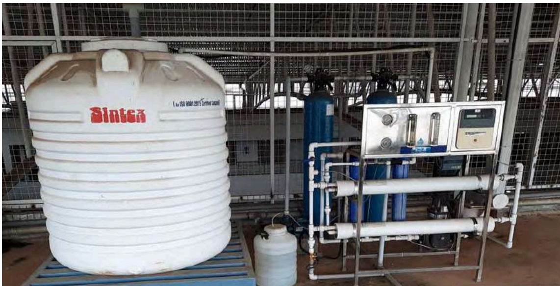
Reverse Osmosis (RO) Plant at YIMS
