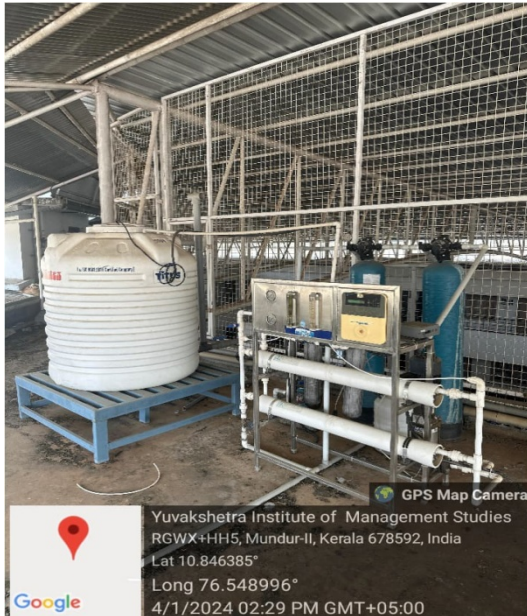
Water Purification System
